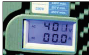
Volts and amps meter control display.
